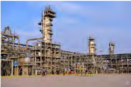
Hawiyah Gas Plant
